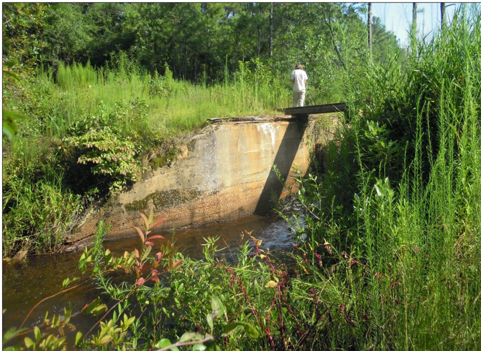
Figure 13. A view of the downstream spillway training wall on the west side of the dam.
