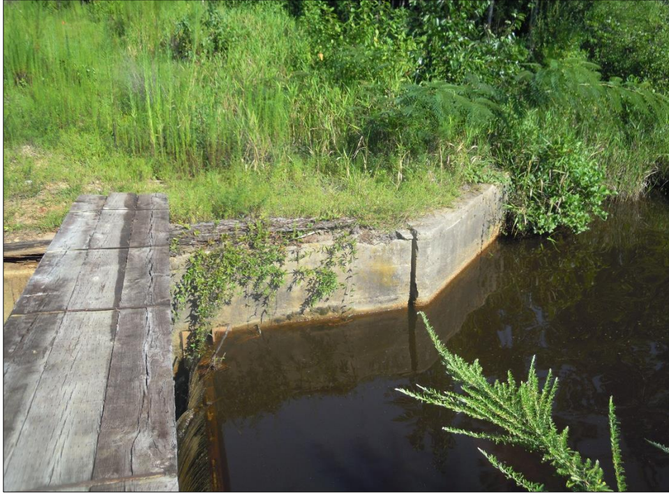
Figure 14. View of the upstream approach wall on the west side of the dam.
