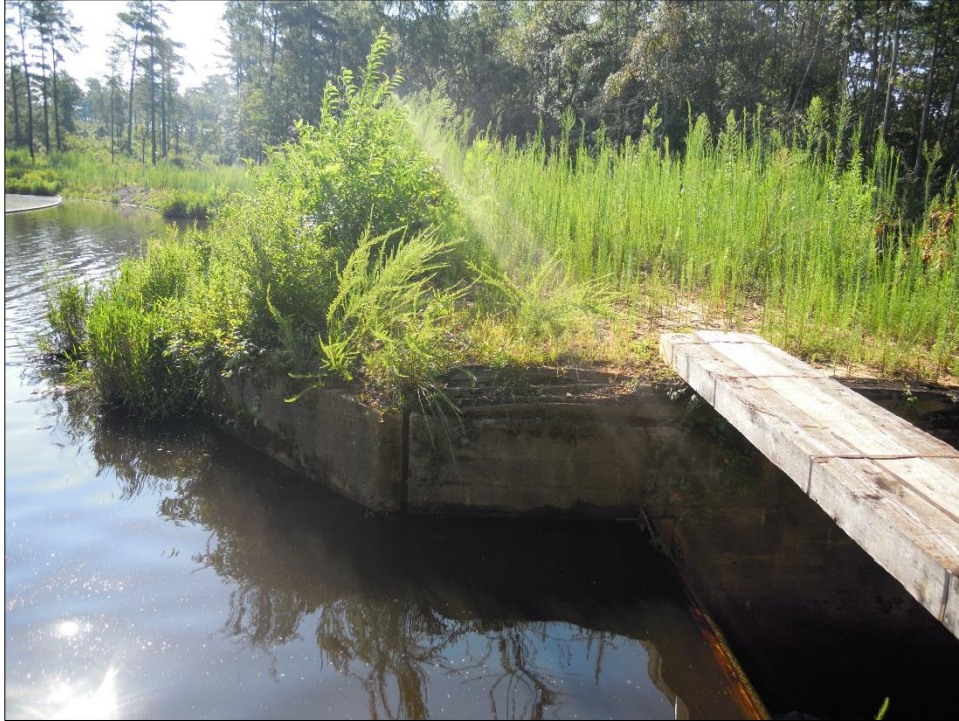
Figure 12. View of the upstream spillway approach wall on the east side of the dam.
