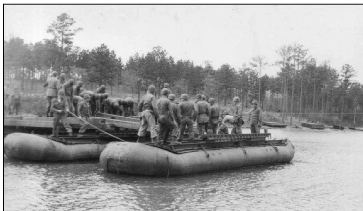
Figure 7. Engineers constructing a bridge across Smith Lake in 1951, NARA College Park, RG 111 SC WWII, Box 212, Photo SC376463. 35
