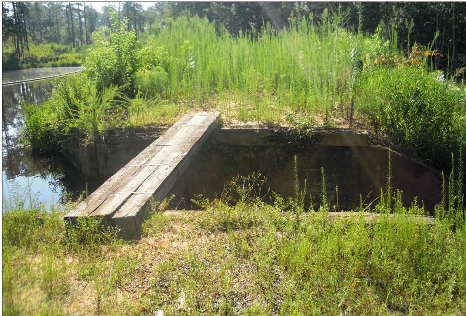
Figure 15. The wood sills running on either side of the dam spillway are all that is left of the wood access deck/bridge that crossed the spillway. It was removed ca. 2014 because of severe rot. The deck likely dated to the post-WWII era.
