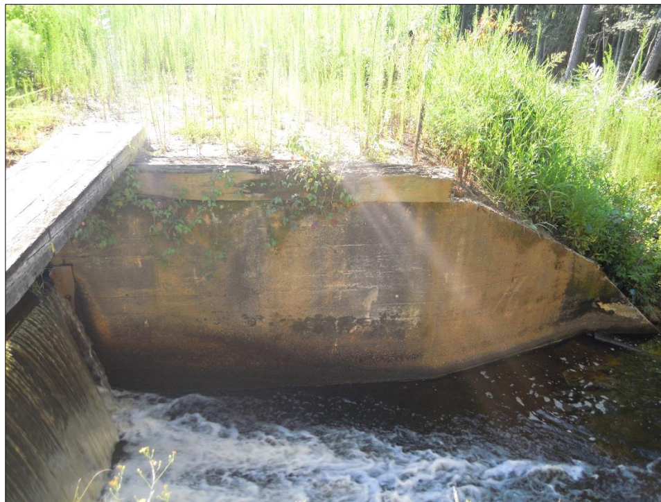
Figure 11. A view of the downstream spillway training wall on the east side of the dam.
